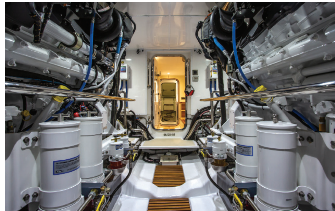
New construction techniques and materials enabled the builder to introduce more volume in the engine room, where headroom is more than 6 feet.
