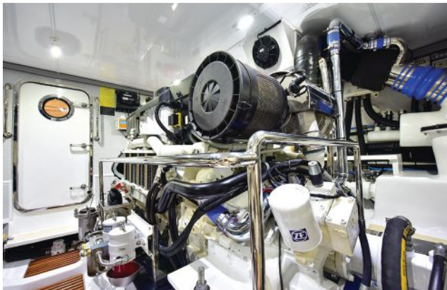
There is lots of space to get to any system in the engine room.
